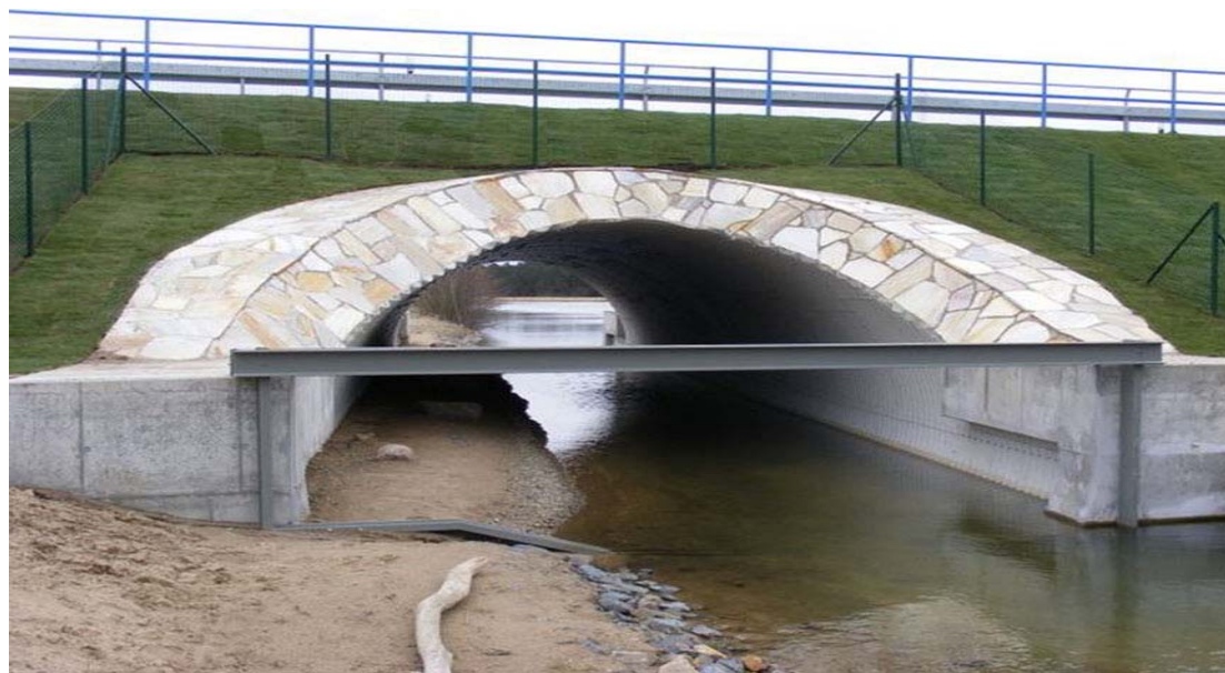
Figure 17: Passage tunnel for otters at the Havel-Oder-Waterway (from: WSA Eberswalde)
